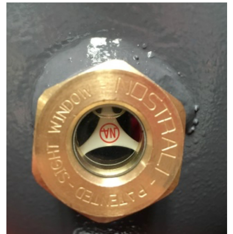
✗ Completely full Tank
