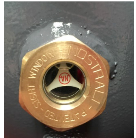
✗ Completely full Tank
